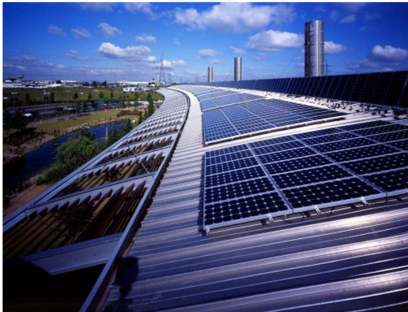
CEME roof-mounted photovoltaic array
