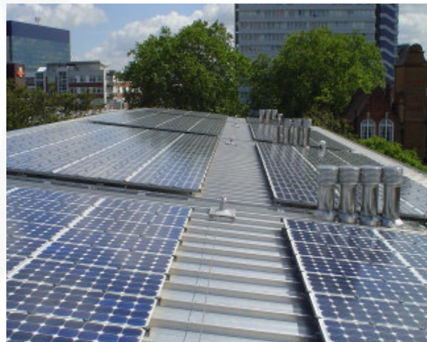
Roof-top photovoltaics (© WBP).
